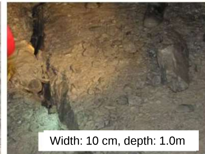
Tunnel floor Fractured
