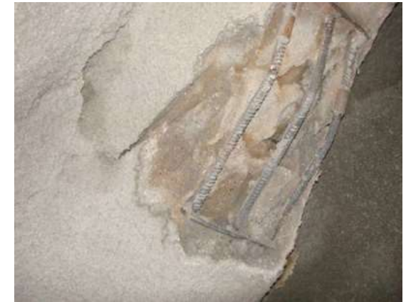
Fall of sprayed concrete
