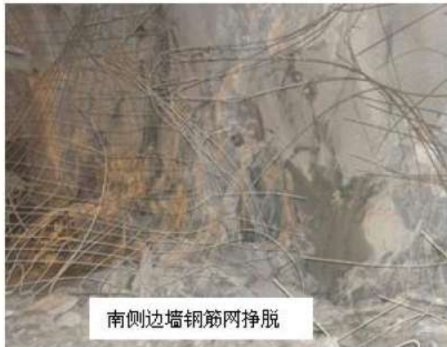
Steel mesh destroyed
